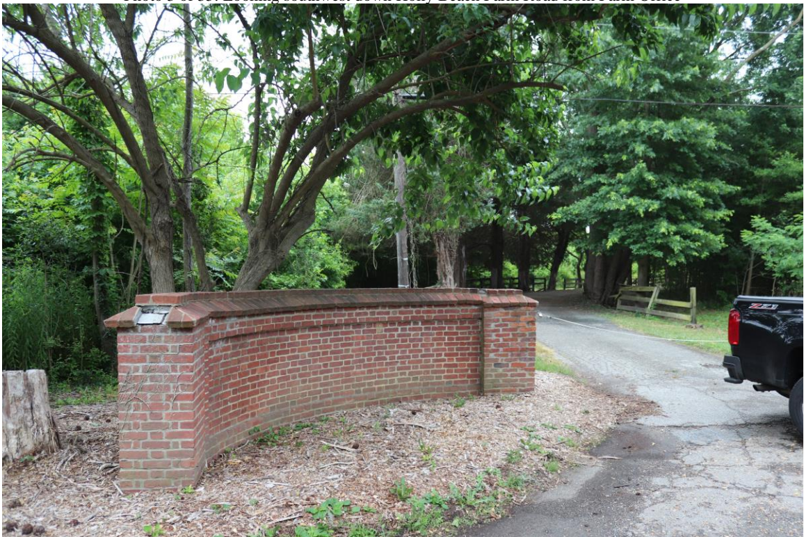
Photo 4 of 35: 1917 Holly Beach Farm Road, gate on Holly Beach Road to the stable complex, looking east
