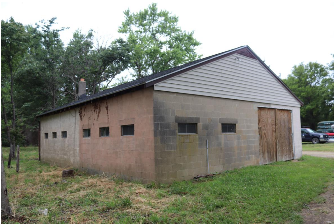
Photo 11 of 35: 1801 Holly Beach Farm Road, Workshop, southwest elevation and northeast façade, looking northeast
