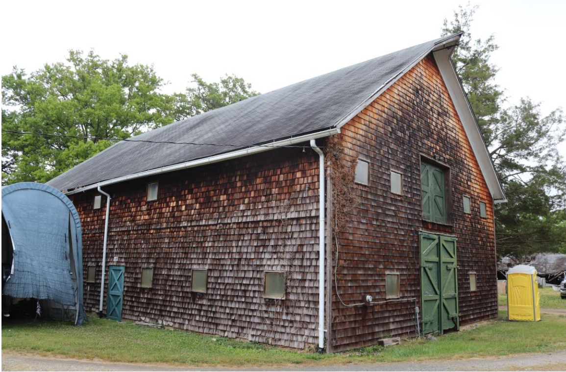
Photo 7 of 35: 1801 Holly Beach Farm Road, Rectangular Stable, northwest elevation and southwest Façade, looking northeast
