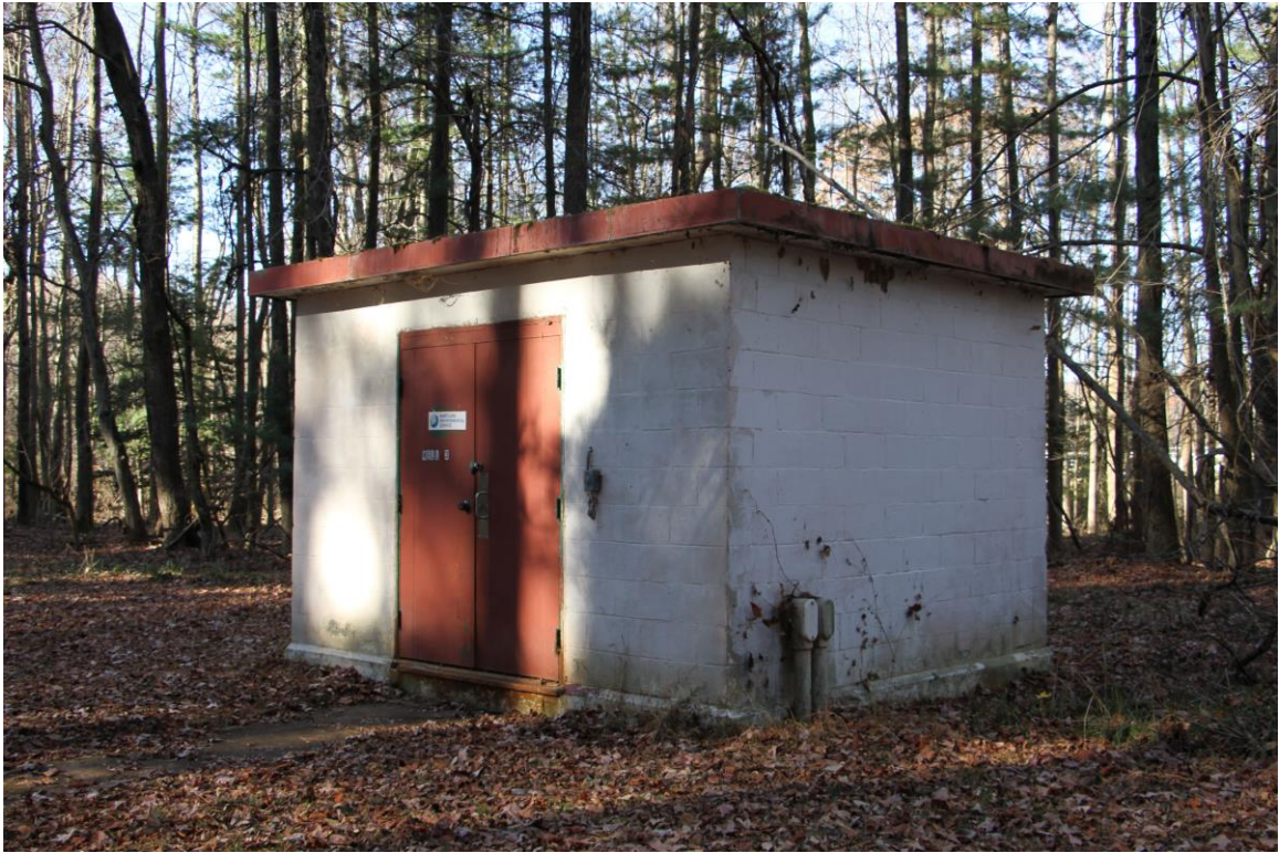
Photo 19 of 39: East College Parkway Area, Well House No. 3, south façade and east elevation, looking northwest
